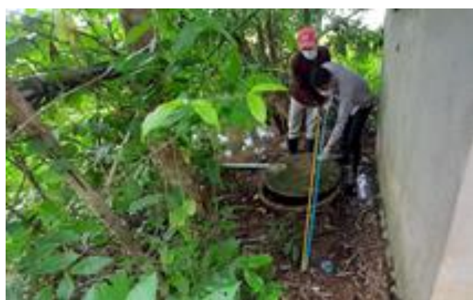
Figure 3: Measuring if a second pit can fit next to the existing pit to create an alternating dual-pit latrine
